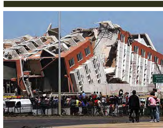
A collapsed residential building in Conception reflects the devastation of the Chile earthquake.
