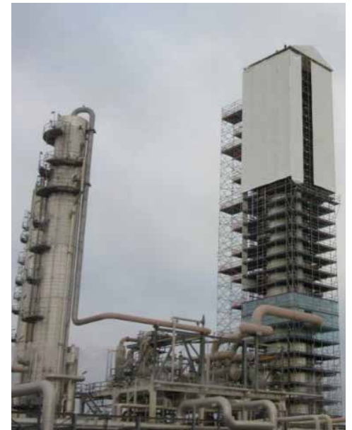
Scaffolding around a distillation tower is smothered by a re-usable curtain wrap.
