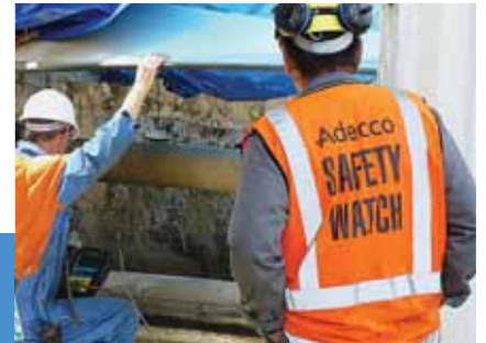
A Safety Watch contractor observes a worker during Methanex's Waitara Valley plant turnaround.
