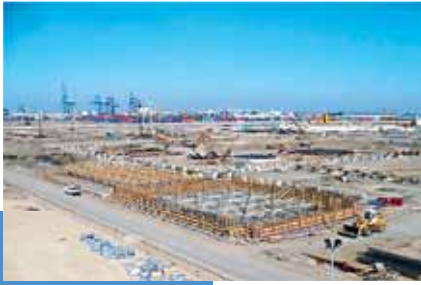
Ongoing construction at Methanex's Egypt methanol project. The plant is scheduled for start-up in early 2010.
